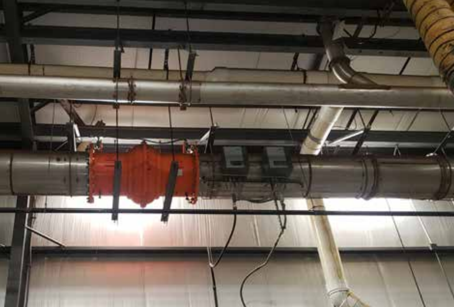
LEFT: Vidimos installs fume collection systems like these for industrial clients in Indiana.
