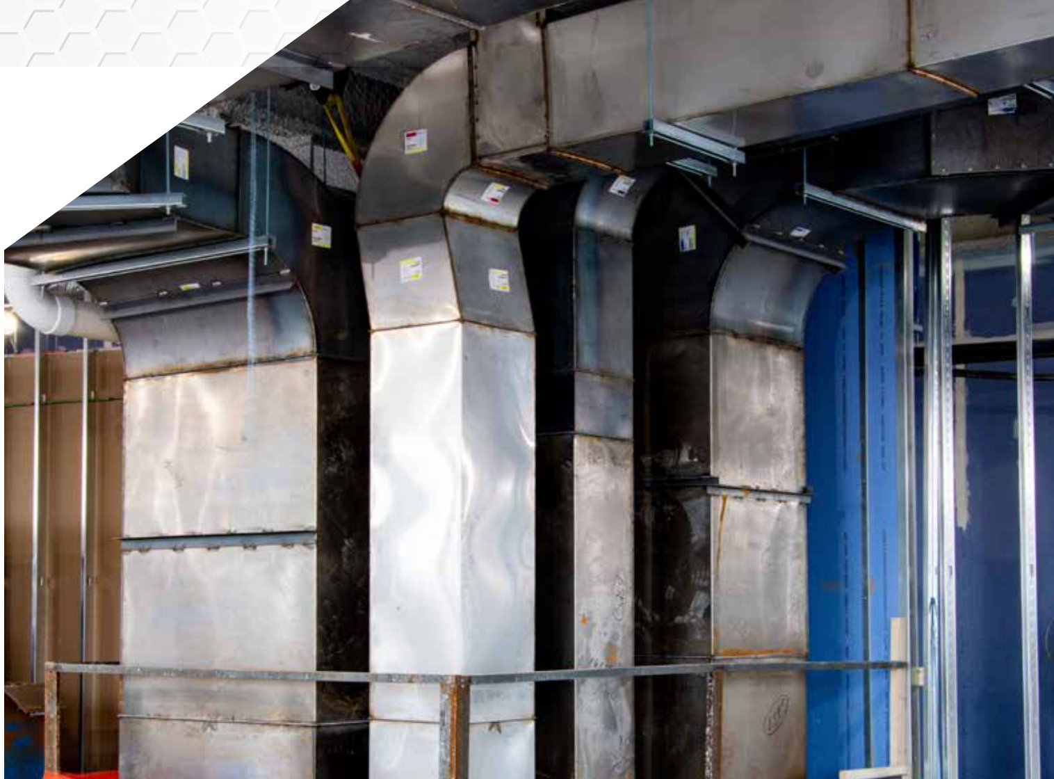
An estimated 70% of the sheet metal work for the MetroHealth Transformation project was done via prefabrication. A work area was set up onsite to pound out the duct work and put it together.
