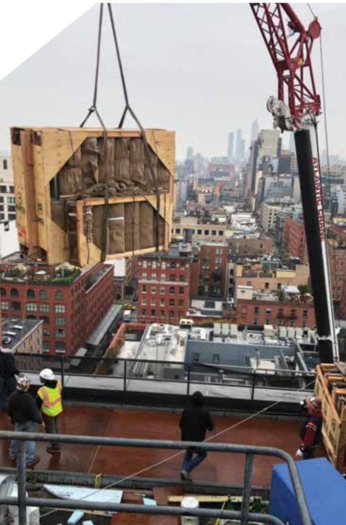
FAR LEFT: A bird's-eye view of the cooling tower. ASMF constructed and installed aluminum guardrails around the perimeter of the roof, along with a site screen wall to conceal the cooling towers.
