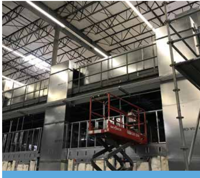
Installation progress of return duct risers, serving cleanrooms, connecting to mechanical mezzanine above.
